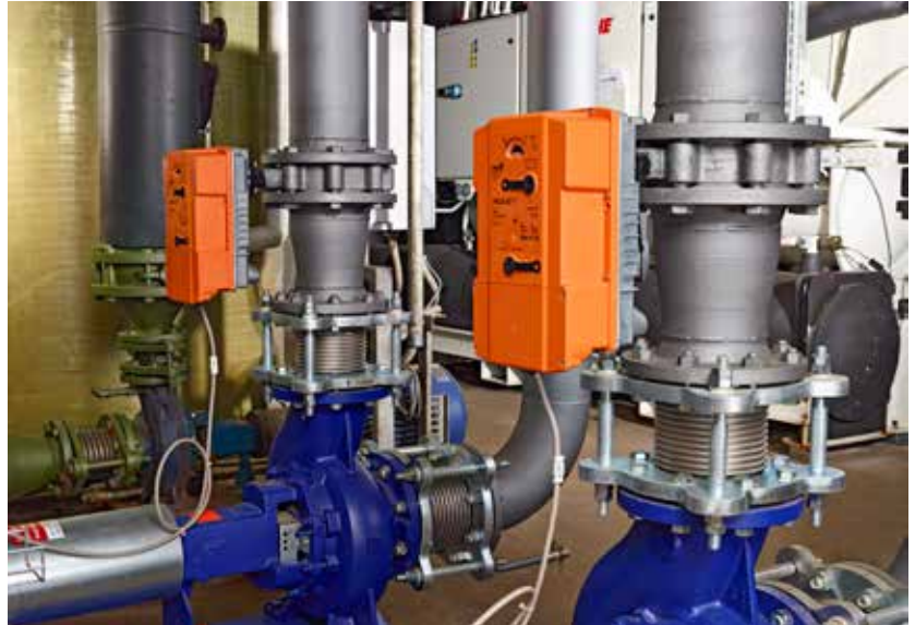
The innovative PR actuator installed in the new plant of Kuhn Champignon AG.
